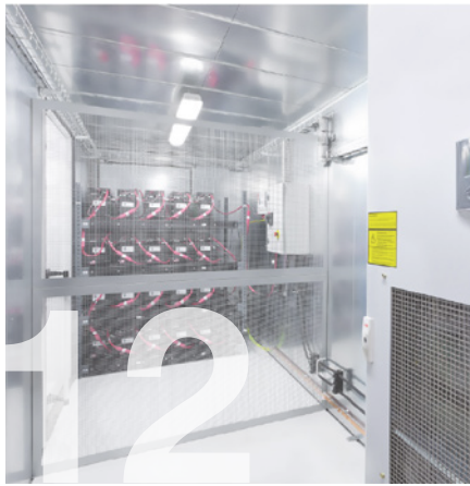
Battery Energy Storage Systems
